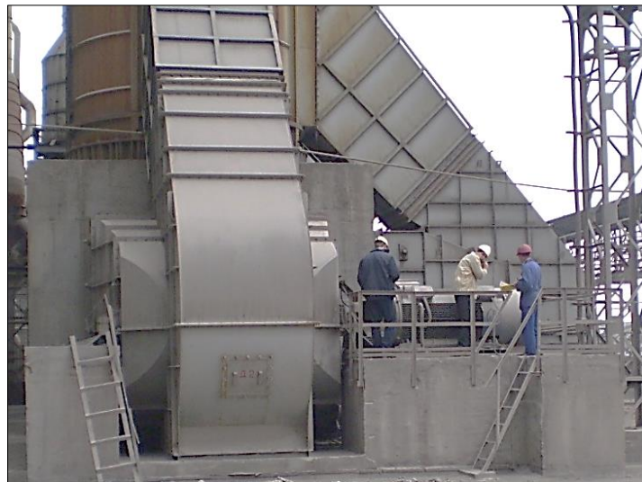
Fig. 1: General view of the induced draft fan of the gas cleaning unit in the electric steelmaking shop
